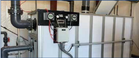
Radon removal and pH Adjustment at 160 GPM
